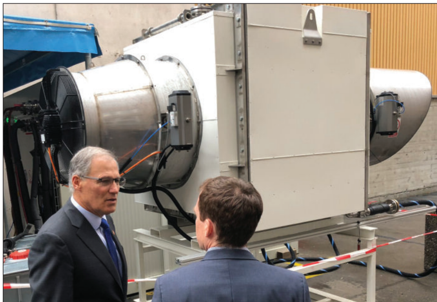
A Climeworks DAC unit in Switzerland Photo by Jay Inslee via Flickr
